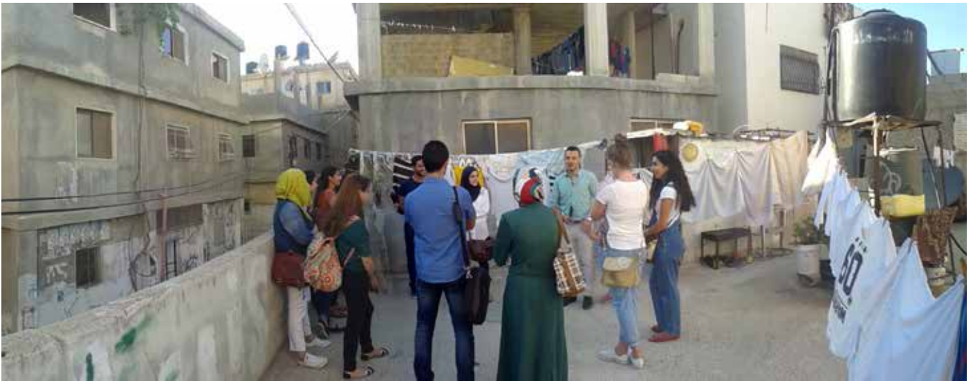
Figure 7 A view from Mahmoud's rooftop before the start of the construction works.
